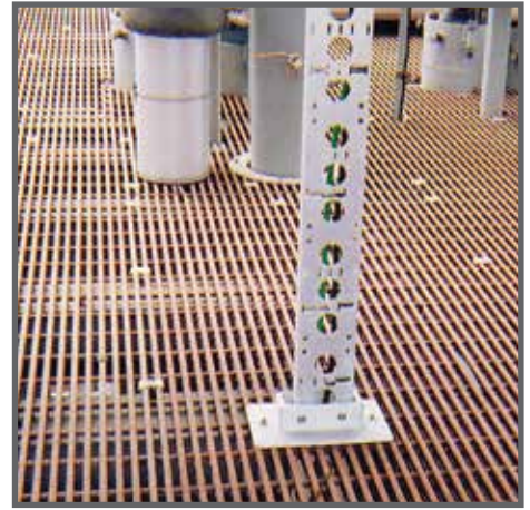
Offshore Oil & Gas Platform
